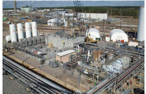
Modular Caustic Side Solvent Extraction Unit (MCU)
